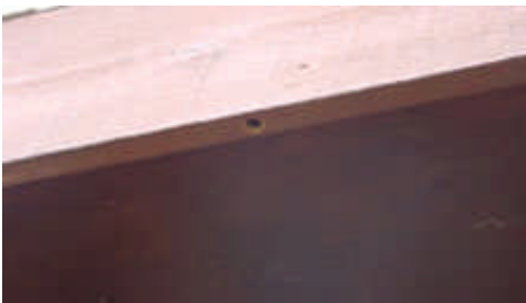
Figure 2. Carpenter bee entrance exposed in wood.
