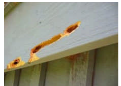
Figure 4. Carpenter bee gallery siding below the fascia.
